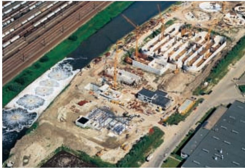
Antwerp-South is currently being renovated in order to comply with the effluent standards.
