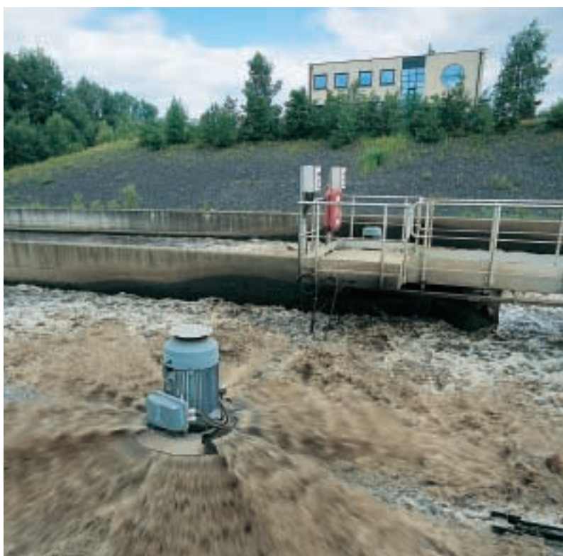
Houthalen WWTP. In 2002 a new form of control was introduced based on on-line measurement.
