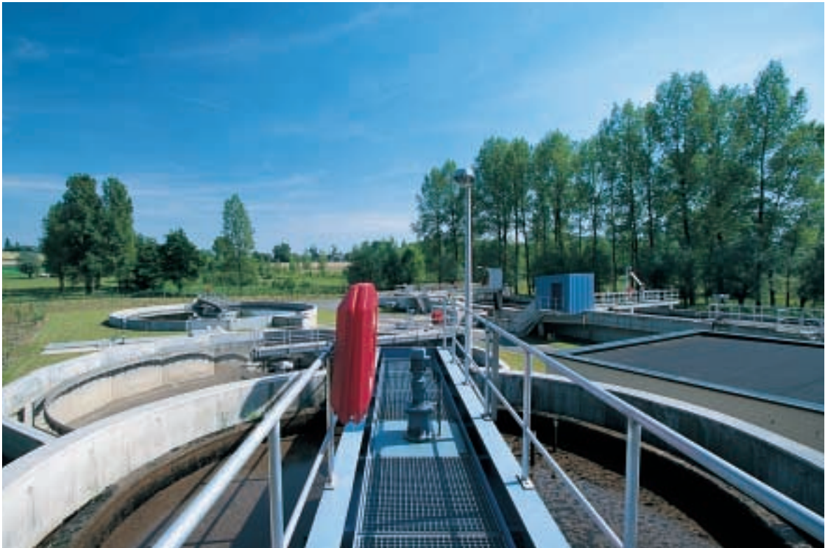
Brakel WWTP is located in VEN area and in a nature reserve.
