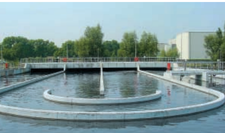
Aeration basin at Merelbeke WWTP.
