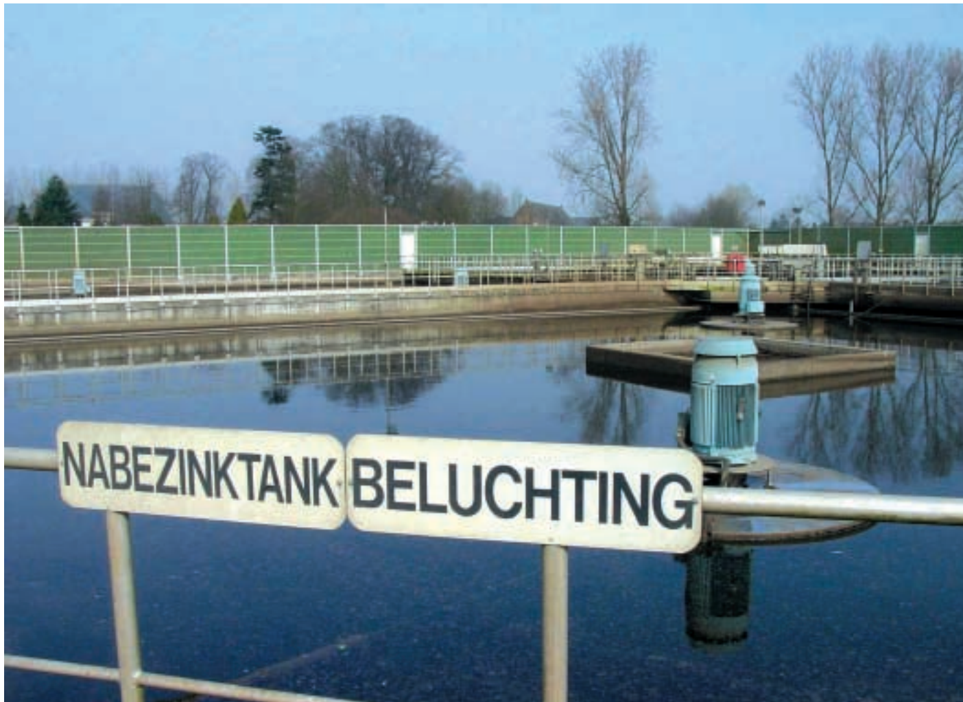
Geraardsbergen WWTP. In the background: our very own 'wall of Geraardsbergen'.
