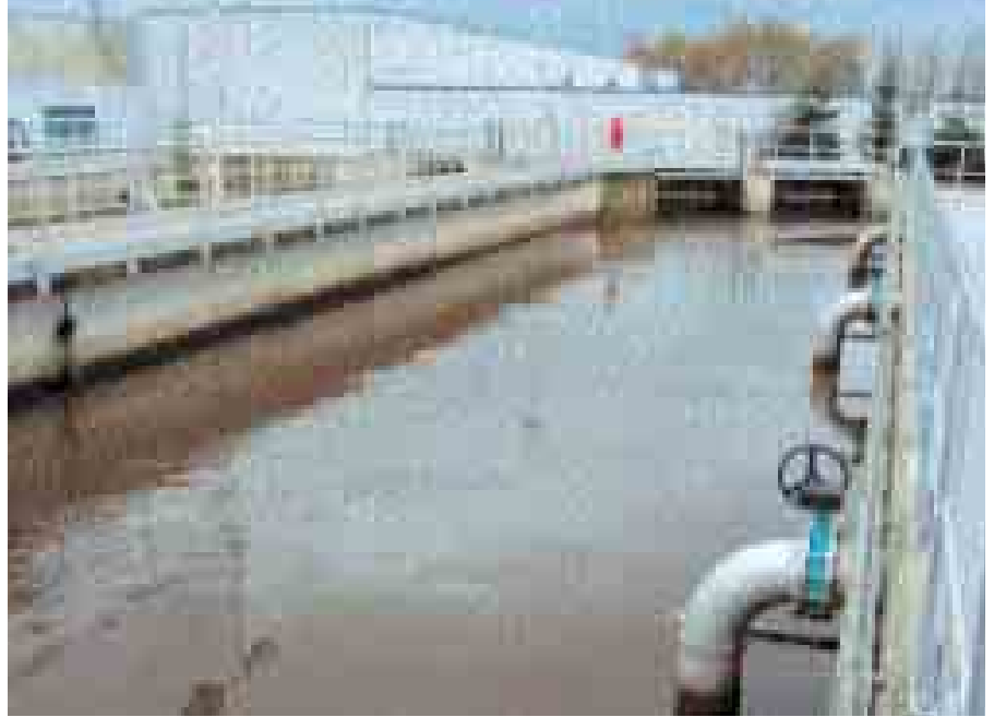
Turnhout WWTP aeration basin. The nitrogen standard was achieved for the first time following the renovation in 2001.
