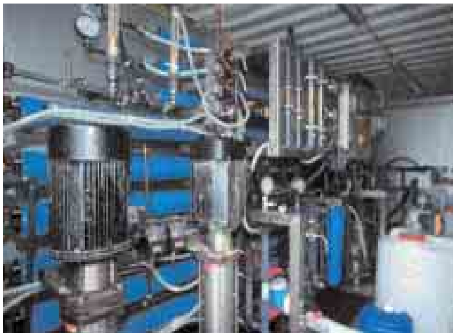
Test setup for reverse osmosis in Waregem.
