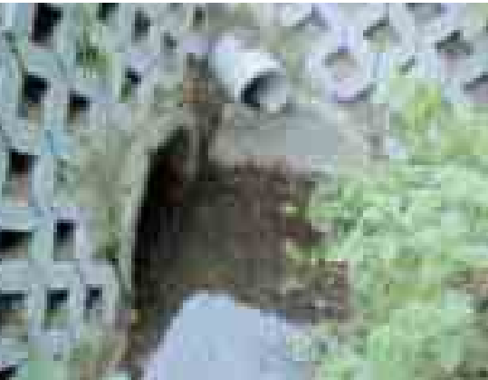
An inlet to the Millebeek in Zekegem was bricked up.
