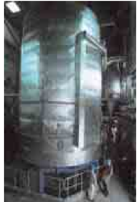
Sludge dryer in Bruges.
