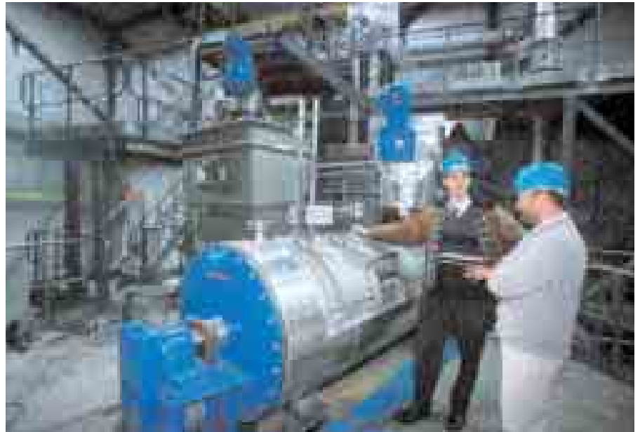
The mixing installation on top of the sludge dryer in Bruges.
