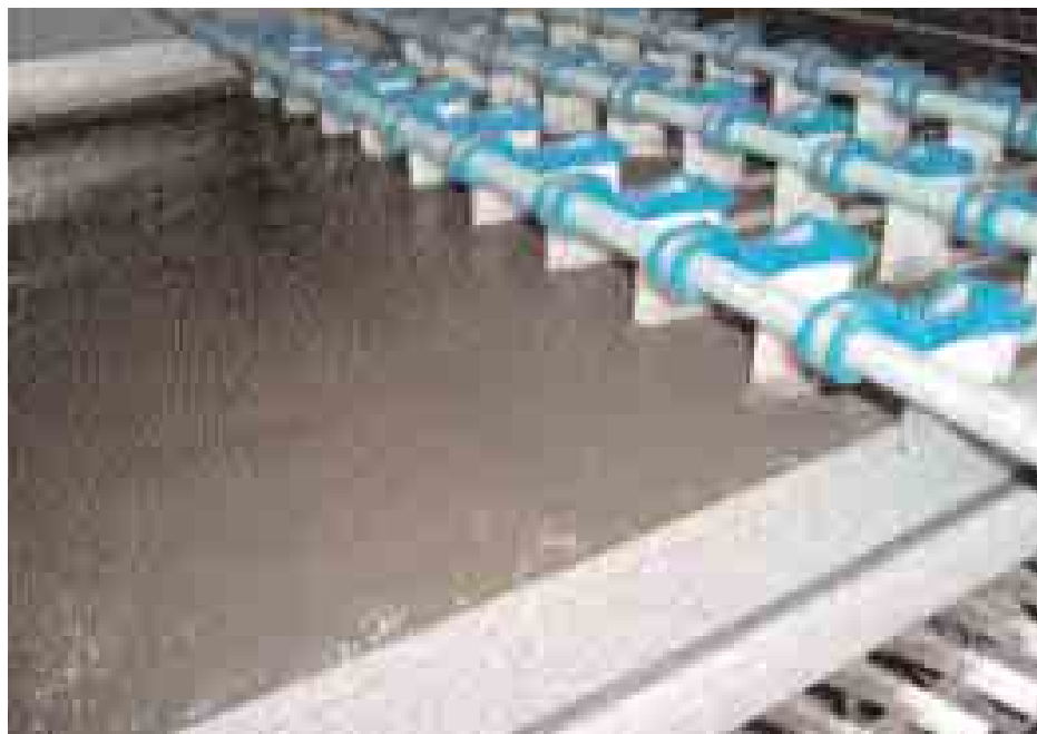
Sludge thickening table at Menen WWTP.
