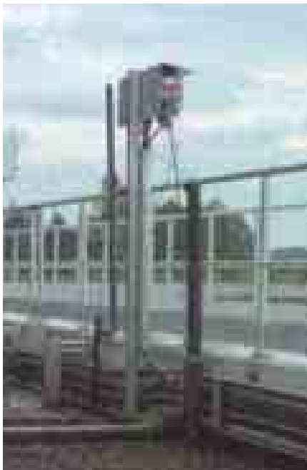
An oxygen meter measures the concentration of dissolved oxygen in the aeration basin.
