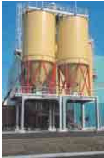
Sludge dryer in Houthalen. Sludge silos in the foreground.
